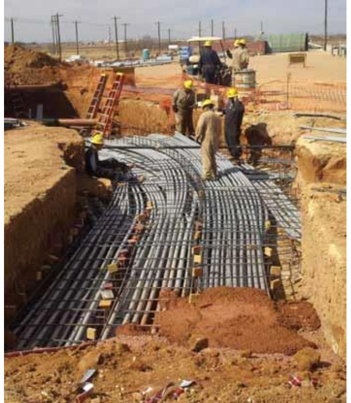
Wide duct bank being excavated/installed in a congested gas plant in West Texas.
