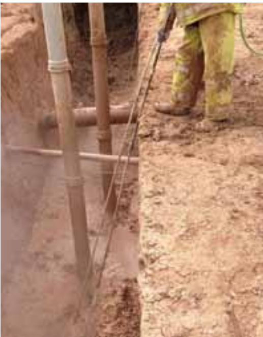
Hydrovac has become the standard for excavation work inside gas and electric facilities (Texas).
